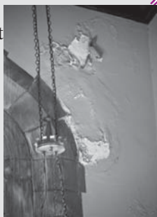
Repairing peeling plaster in the sanctuary will be one of the projects in the sanctuary construction project in 2011.
